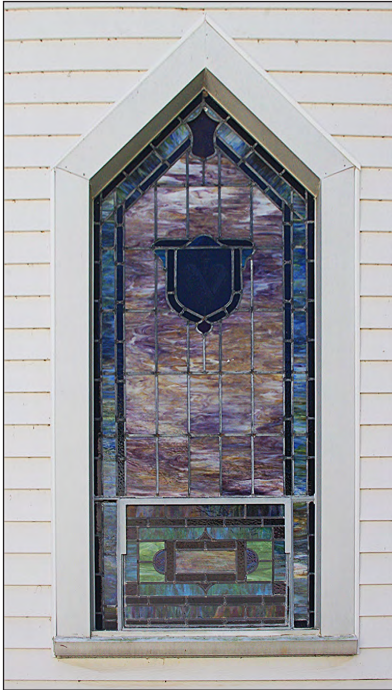
PLATE 36: Stained-glass Window Detail, West Elevation, Mizpah United Methodist Church (RK1452), Rockingham County, North Carolina
